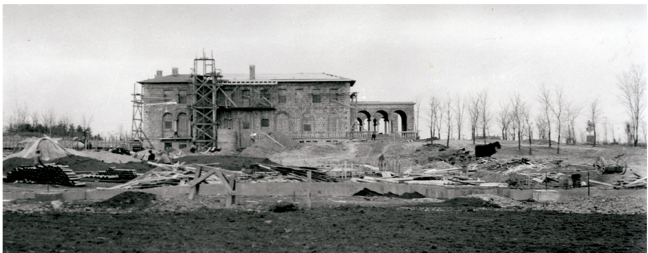
The Samuel Insull residence designed by Benjamin Marshall in 1914 under construction. Later to become the Cuneo Mansion.
